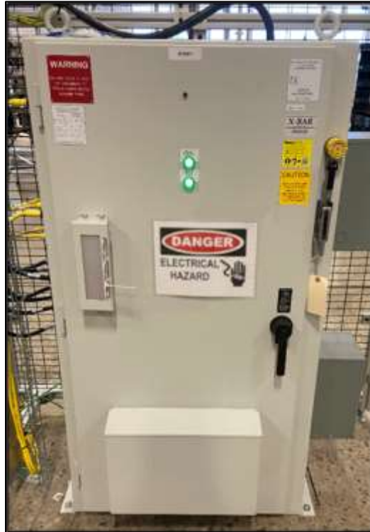
Figure 4-8. An Example of a Power Distribution Panel.
