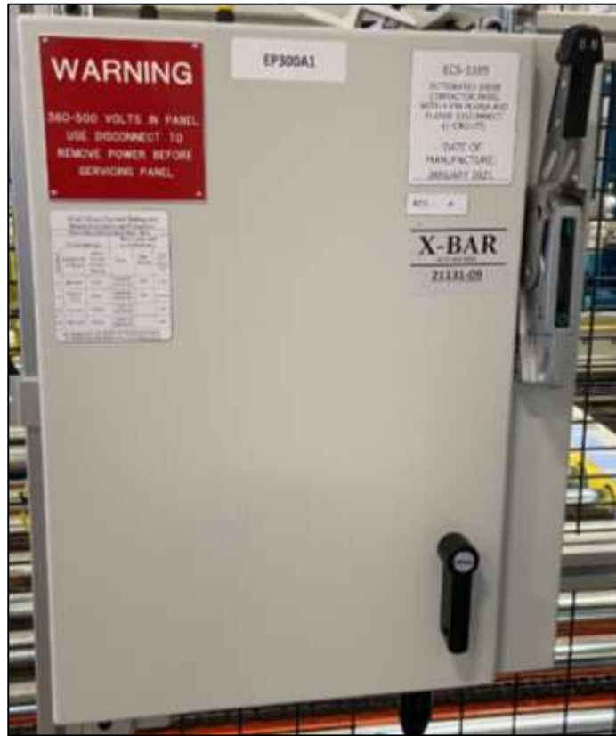
Figure 4-3. An Example of a Conveyor Electrical Disconnect
